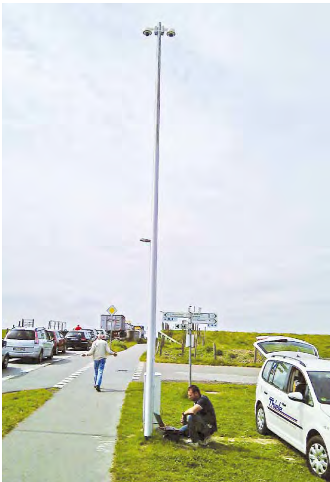
Thiele Hauselectronic Employees Are Setting Up the IP Solution.
